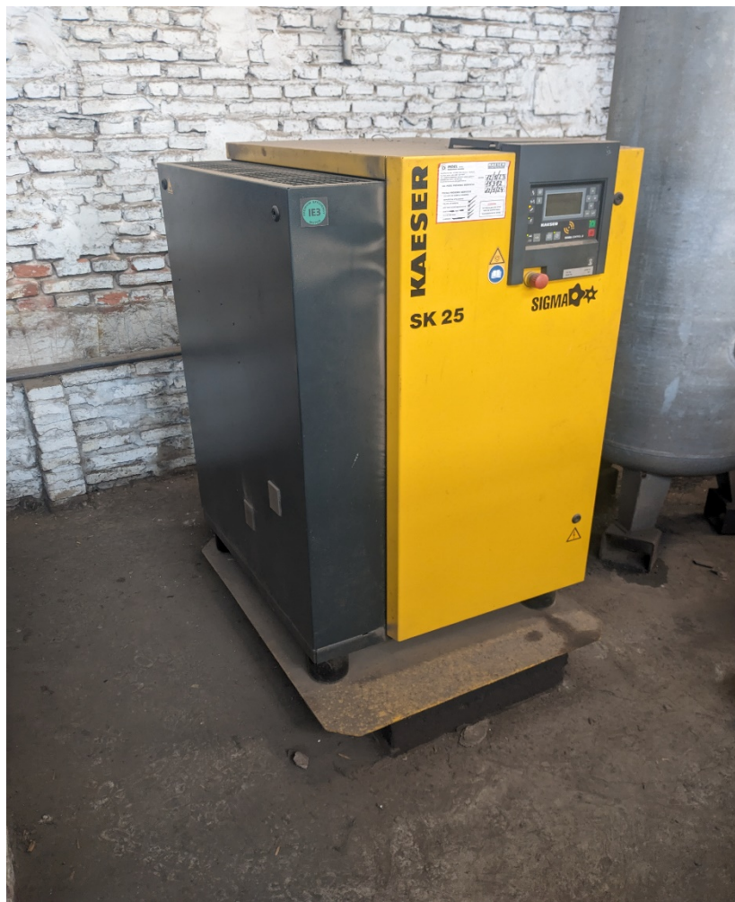
Figura 2. 7 Compresor Kaeser SK 25
